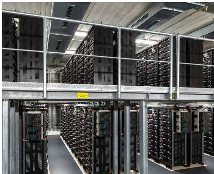
Battery storage in Schwerin: view inside the battery hall. Picture: WEMAG AG
